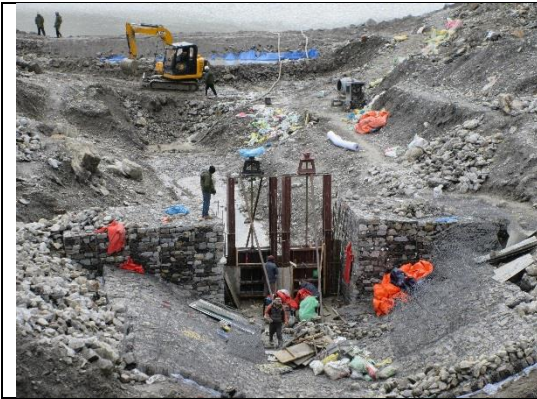
Overview of Imja Lake lowering construction work (foreground – d/s of open channel, background – u/s channel and cofferdam and gate structure).
