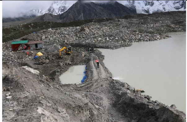
Coffer dam and seepage pond (left) where warehouse and diversion channel are seen in the background.
