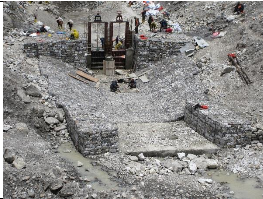
Open channel section at the downstream. The boulder cabling work shall be undertaken before releasing water to existing river section.
