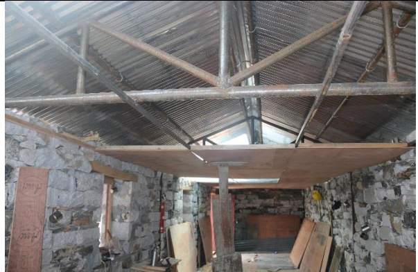
Interior of the office building, the planking of ceiling and walls are ongoing for insulation at high mountains.
