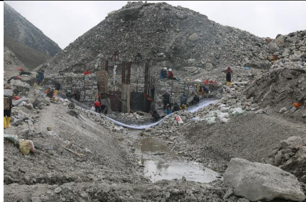
Open channel section at upstream and gabion boxes are being laid over (looking downstream).
