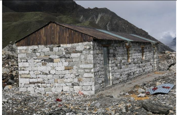
Office building, the roof is in the process of being painted green as per the SNP guidelines.
